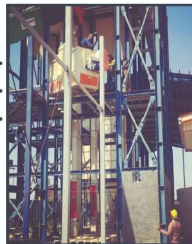
Factory Installation and Commissioning
